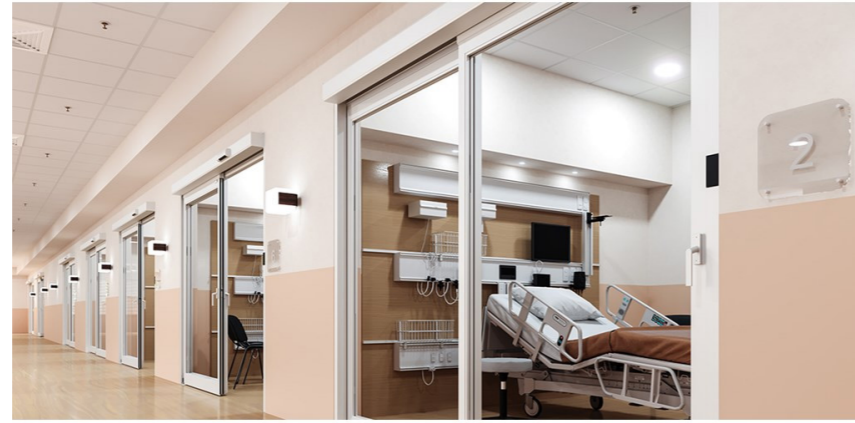
Touchless ICU Doors
