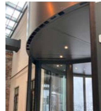
Horizontal air curtain with diffuser integrated in the canopy
